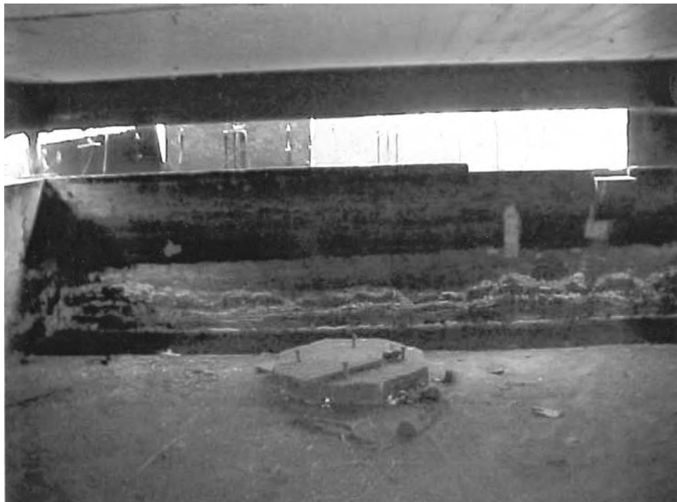
Interior of the BCS showing CRF mounting pier
